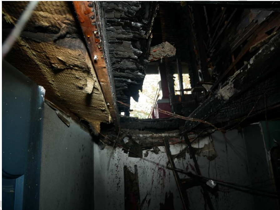
Exhibit 3: Basement view, facing south, looking up to where front door was once located. Matrix of wires are in the foreground.
